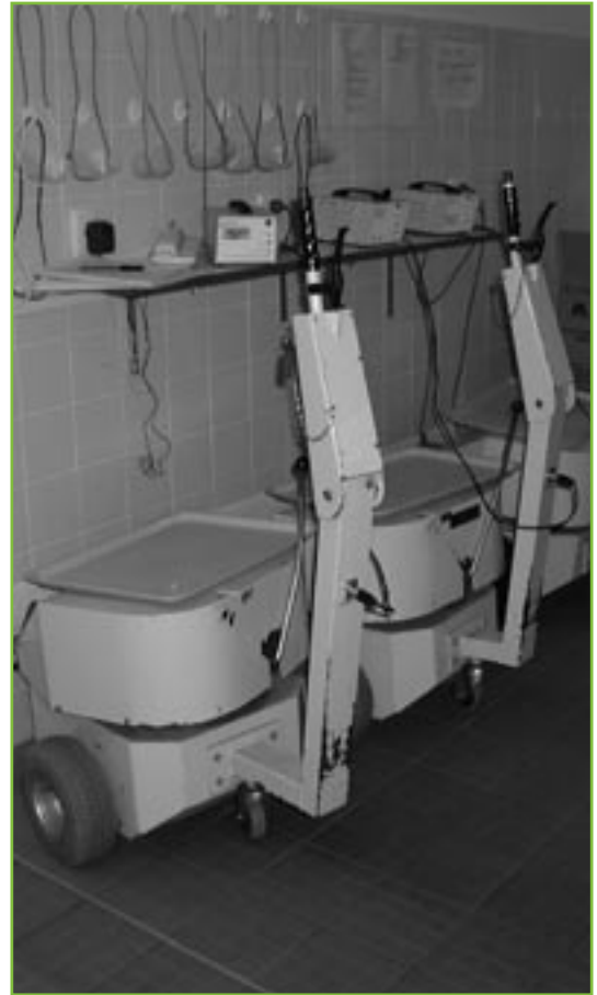
Tow tugs parked in the bay where their batteries are charged
